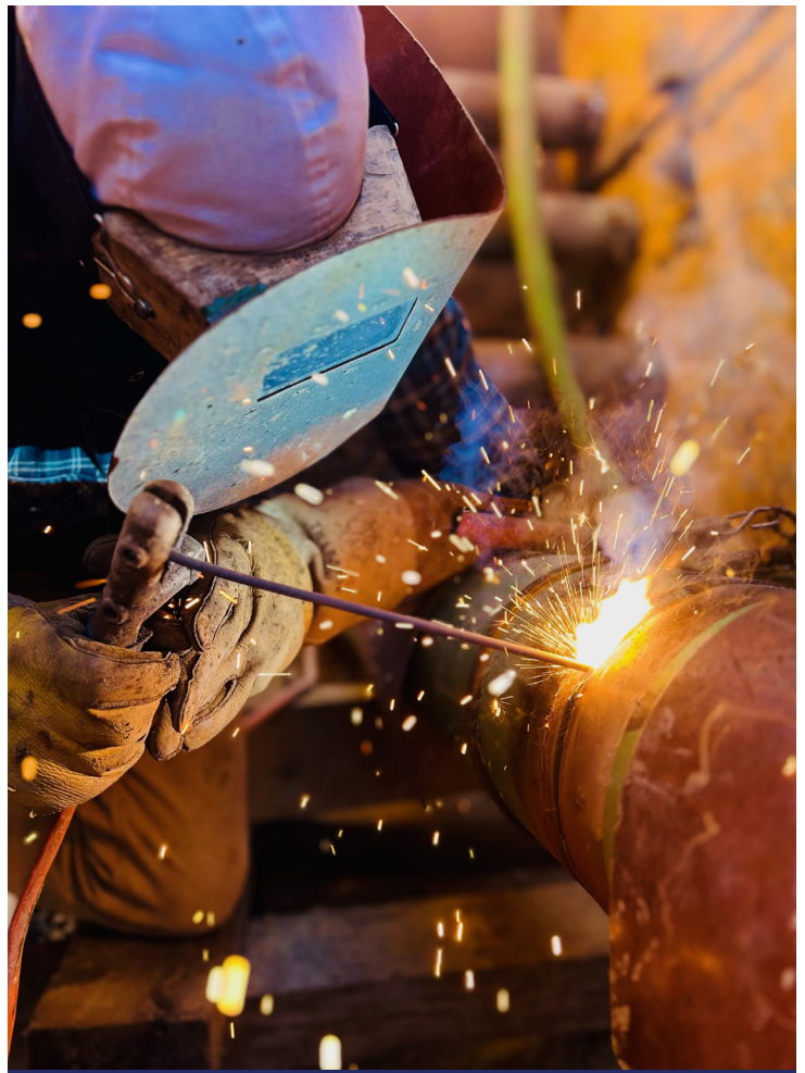
Trevor J. Howerton in Wilson, North Carolina, for B&G Pipeline Company Taken by: Kenneth Rayburn
