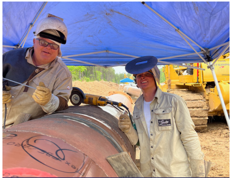
Father and son Darrell N. "Fuzz" Glaze, Jr. and Grant Glaze, third and fourth-generation Pipeliners Local 798 Welder members, welding together on Associated Pipe Line Contractors, Inc., for DTM in Leesville, Louisiana.
