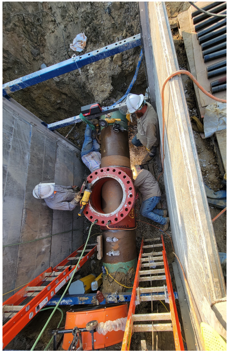
Shane Sheffield, Dakota Taube, Cooper Still, and Ivan Hall for InfraSource Construction, LLC in Erlanger, Kentucky Submitted by: Clark Shaffer
