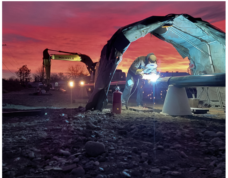
Casey Cazaux for Michels Pipeline, Inc. in Laurel, MT Submitted by: Dakota Dalton
