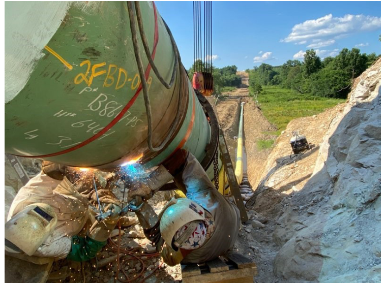
Pictured: Jason Harris and Lee Sloan Buckeye Pipeline, Oak Hill, OH Submitted by: Lee Sloan
