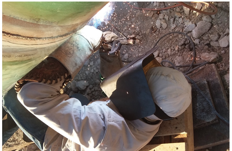
Brandon Williams for Precision Pipeline in Hico, TX Submitted by: Christy Burkheart
